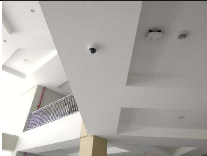
Fire hydrant and light fire extinguisher, CCTV, and gate of UIN Raden Fatah Palembang
