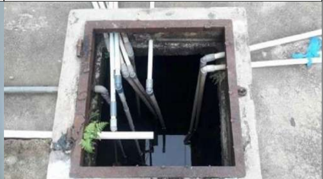
Water Conservation: In Ground Water Tank (UIN Raden Fatah Palembang, Indonesia)
