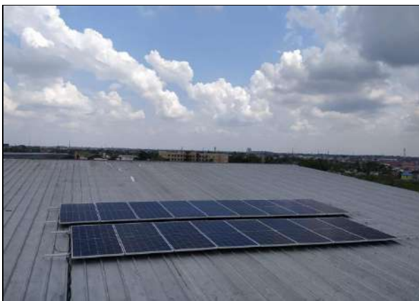
Solar panels on the roof top of the administrative building
