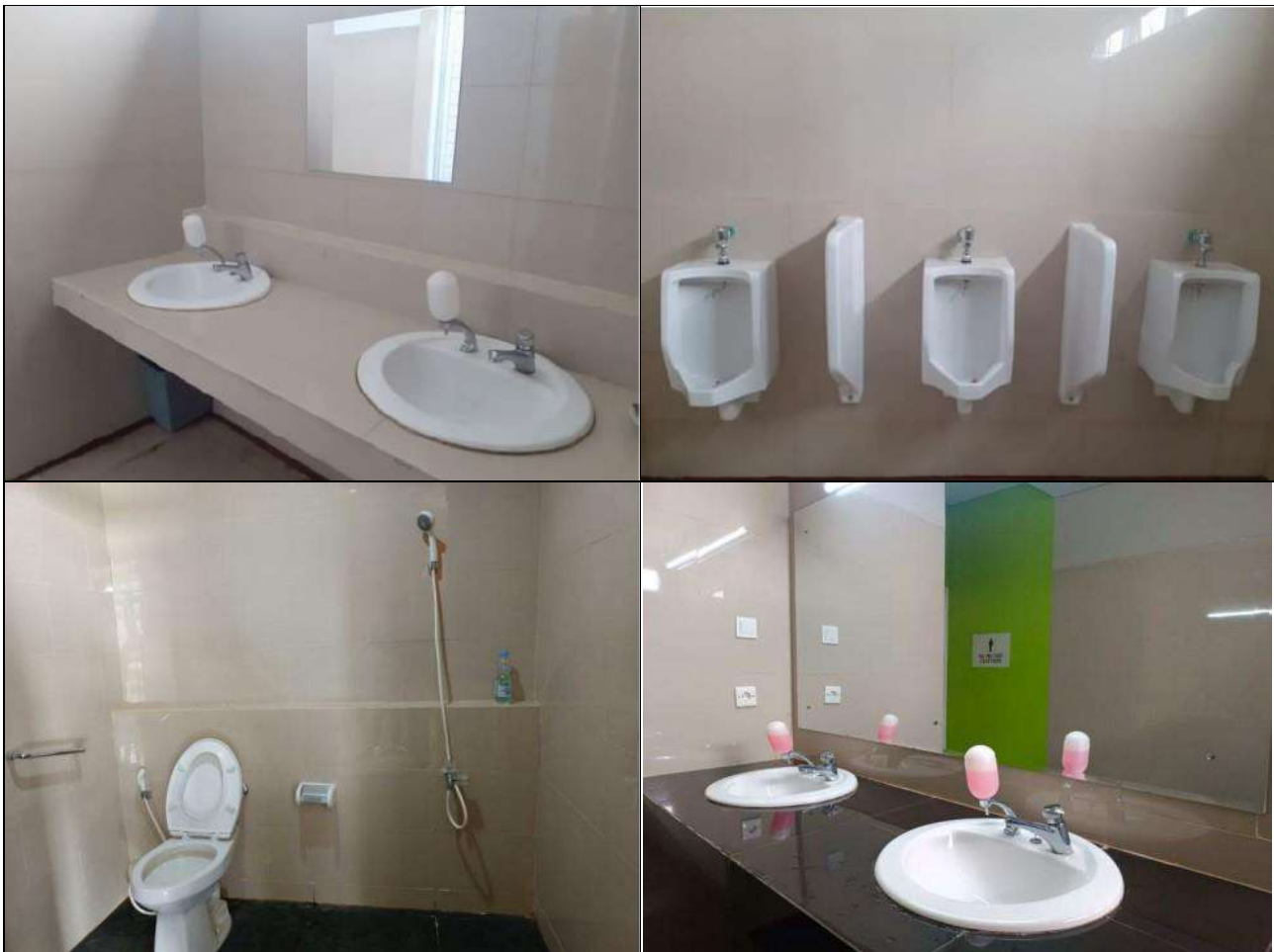
Example of Water Efficient Appliances Usage, include disability access (UIN Raden Fatah Palembang, Indonesia)
